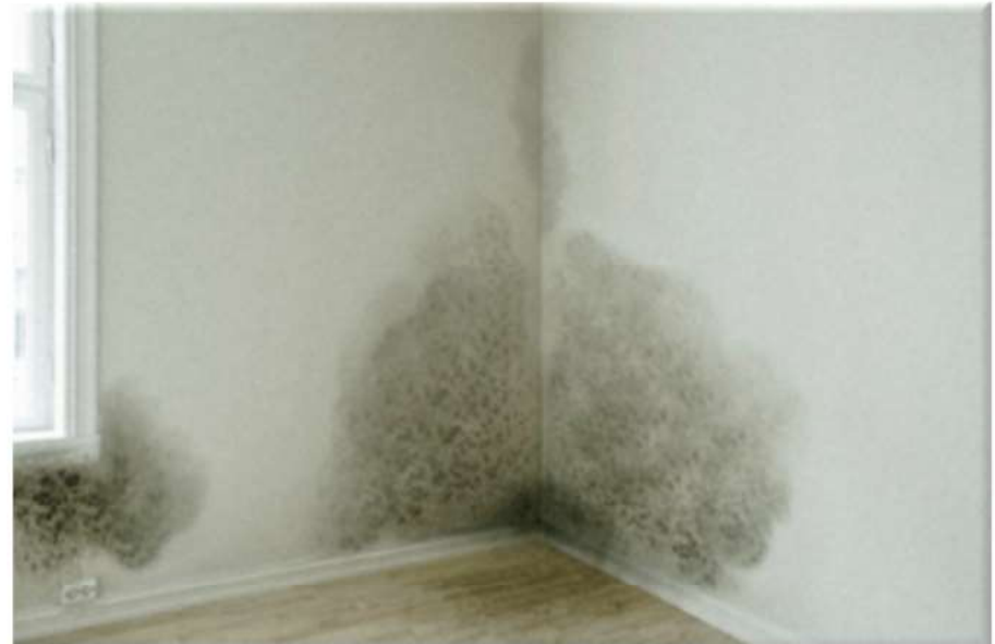
Visible mould in a dwelling
